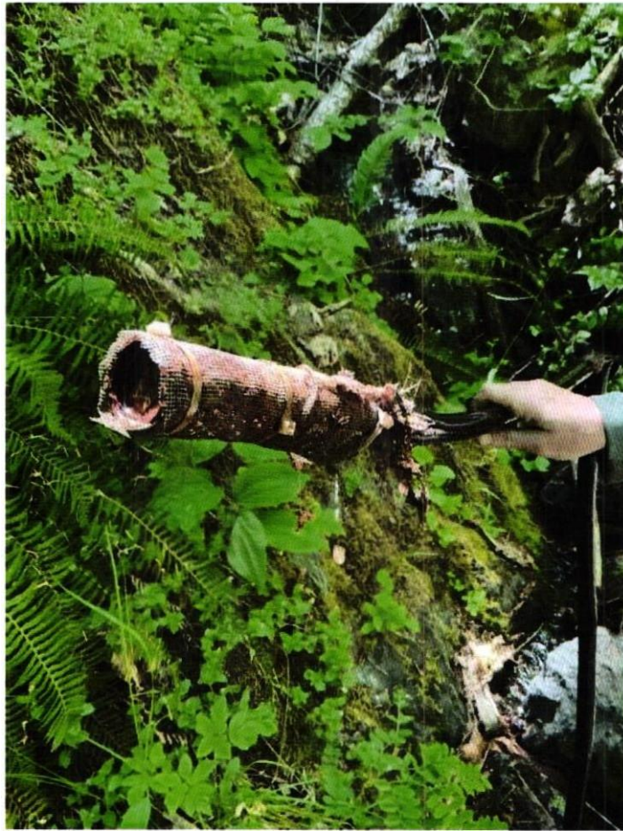
Figure 2. 1602(a) violation includes substantial diversion of the natural flow of an unnamed tributary to Lamb Creek. The photo is of the screened intake for POD 2.
